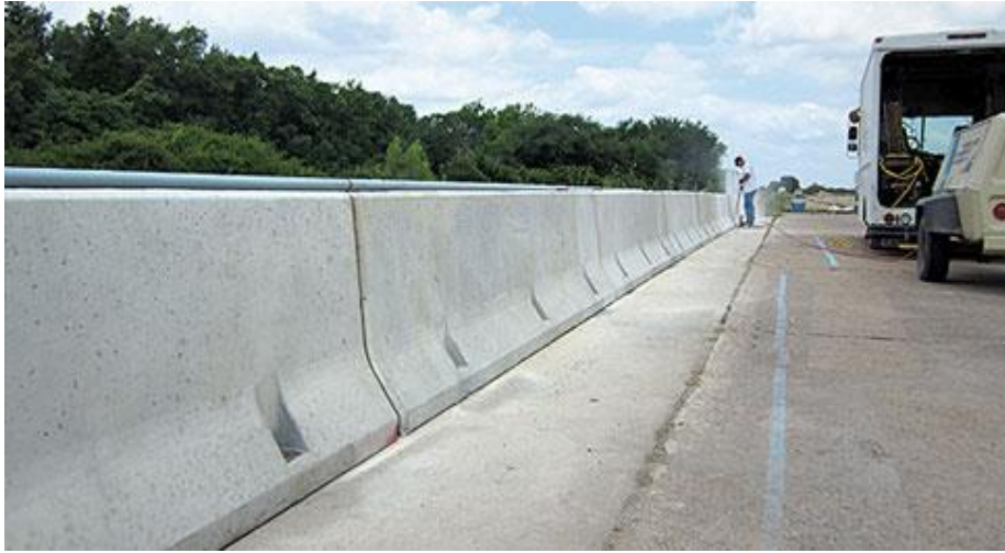
Figure 2- 1. Reinforced Concrete Safety Barrier (Rigid)
